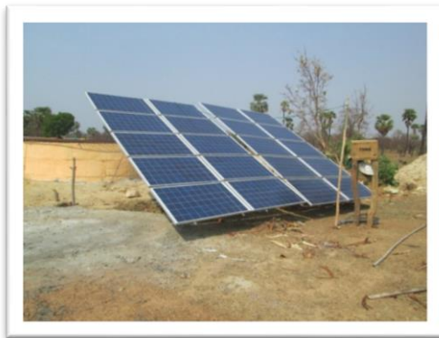
A well with Solar Panel:
